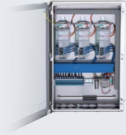
Three FieldConnex FieldBarriers in stainless steel enclosure, ready for commissioning in Zone 1
