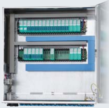
Remote I/O LB in stainless steel enclosure, ready for commissioning in Zone 2
