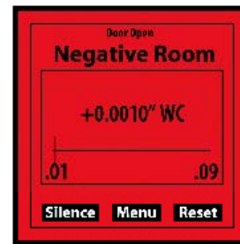
If pressure falls outside of preset limits (Alarmed State), the screen is Red
